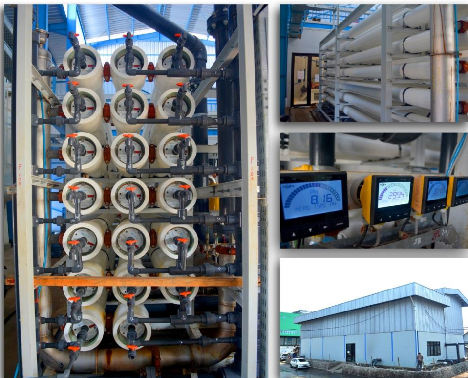
Gambar 2.1 Fasilitas Sea Water Reverse Osmosis (SWRO)
